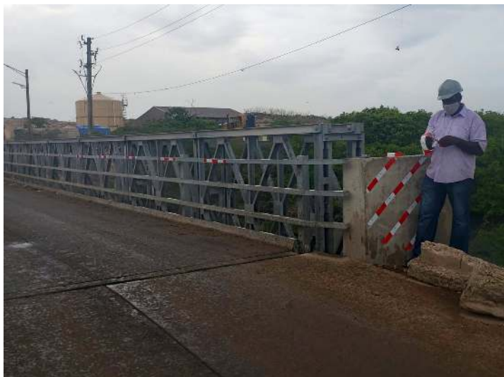
A section of the recently installed Bailey bridge at the Riverton disposal site
